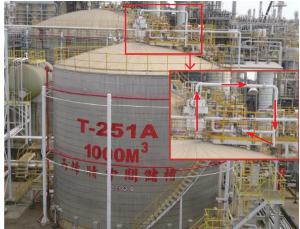
Seal and collect exhaust gas from storage tanks to combustion equipment for treatment
