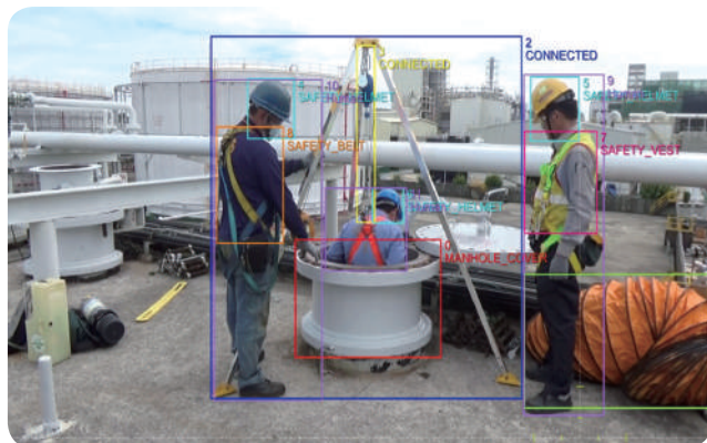
Imaging recognition system for confined space operations in manholes
