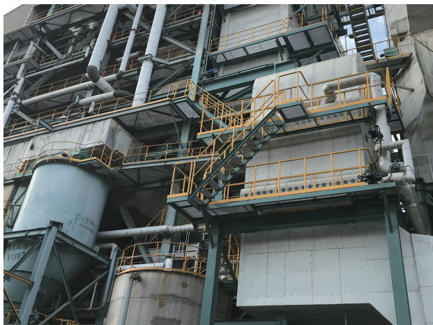
The Control Equipment
