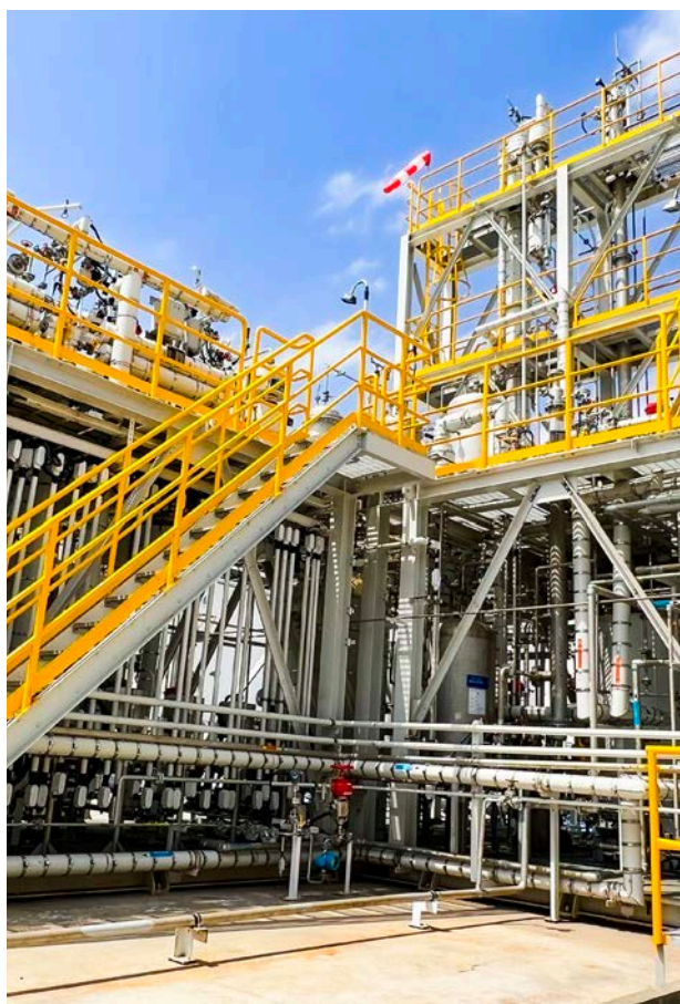
FPC Flue Gas CO 2 Capturing and Utilization Pilot Plant
